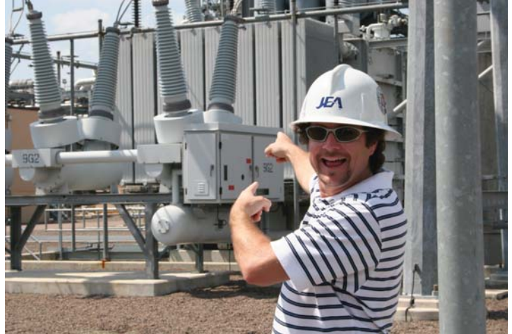
David Reed demonstrates his enthusiasm for saving electricity! Photo taken at Brandy Branch generation station in Baldwin. Those are the step up transformers that take the generated electricity to a high enough voltage to transmit over the large transmission lines.
